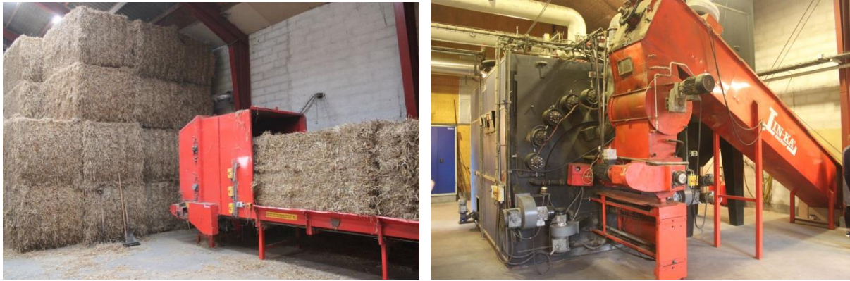
Figure 17: Feeding-unit for straw bales (left) and 1.6 MW straw bale boiler in Ballen-Brundby, Denmark (Source: Rutz D.)
