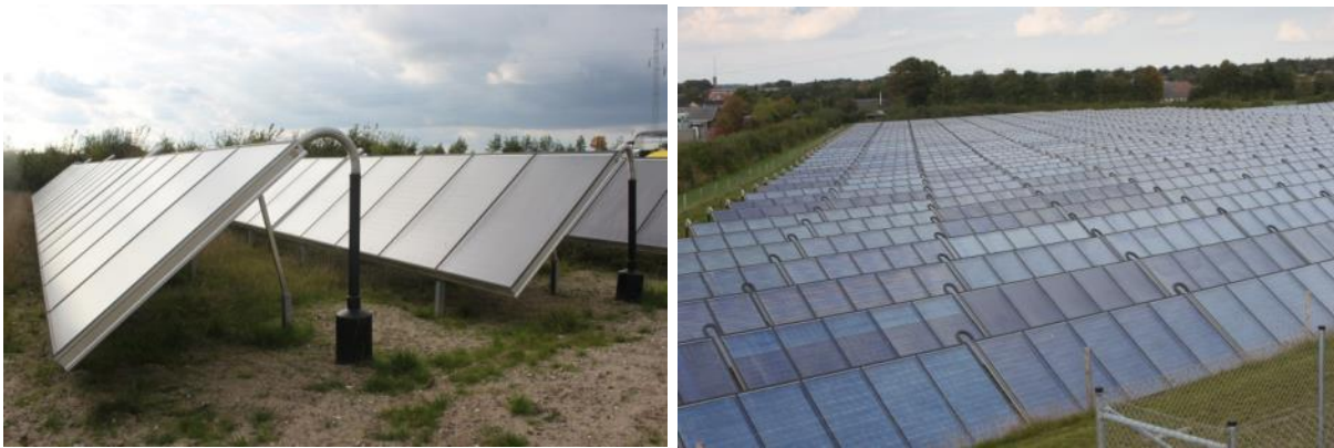
Figure 8: Ground-mounted flat plate collectors of the solar district heating plant in Gram, Denmark (Source: Rutz D.)
