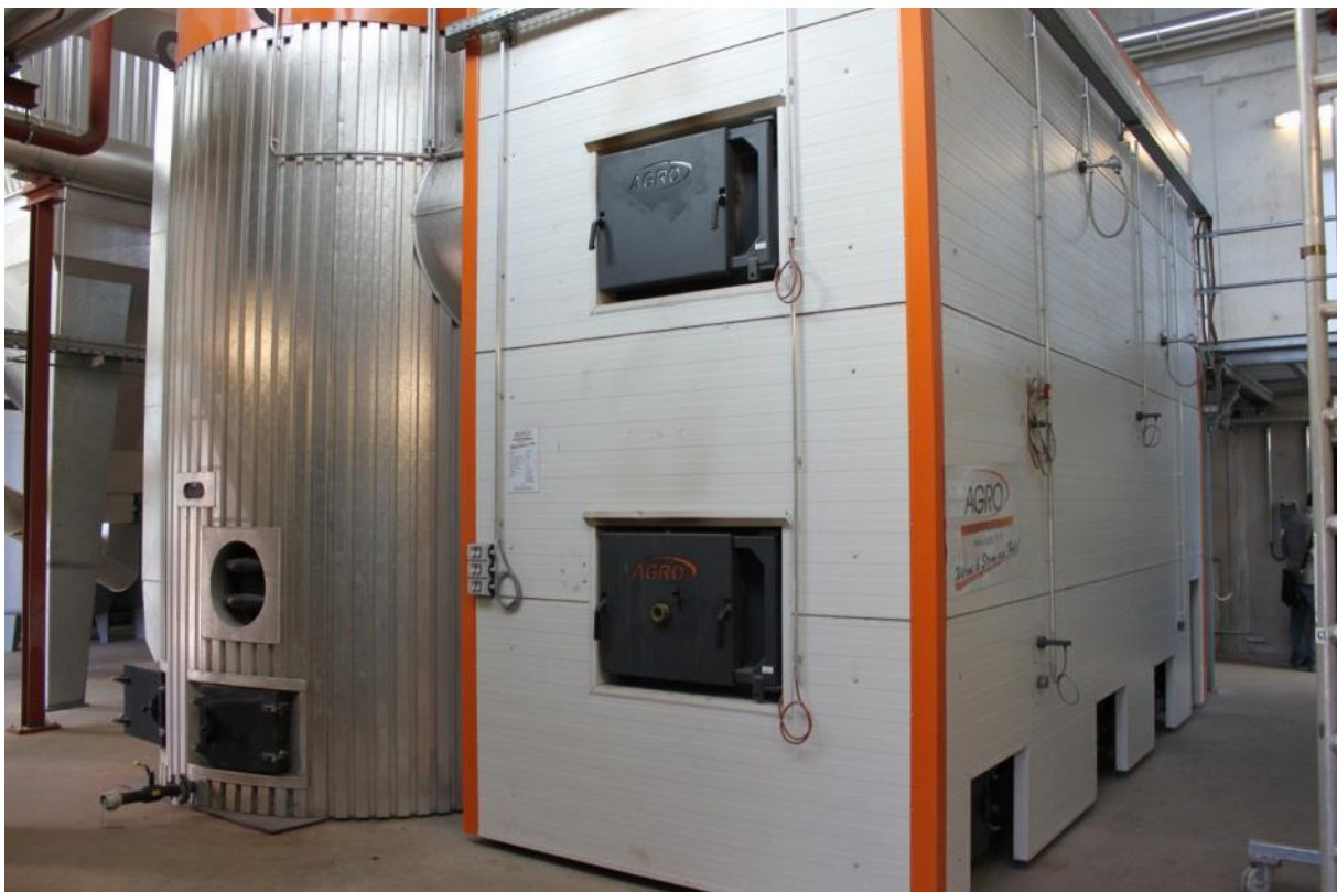
Figure 16: Medium sized woodchip heating system (3,000 kW heat capacity) with the boiler (right) and the buffer tank (left) of the Biomassehof Achental in Germany (Source: Rutz D.)
