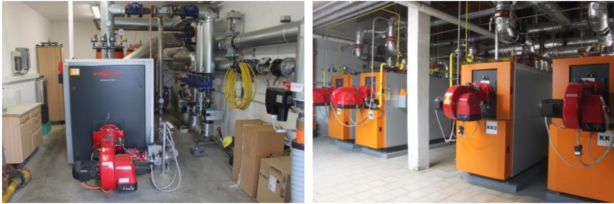
Figure 40: Peak load boiler for fossil heating oil at a biogas plant in Germany (left) and natural gas boilers (right) at a biomass plant in Czech Republic (Source: Rutz D.)
