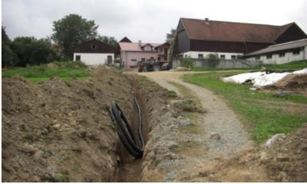
Figure 52: Installation of a heat pipe to the buildings of a farm (Source: Thermaflex Isolierprodukte GmbH)
