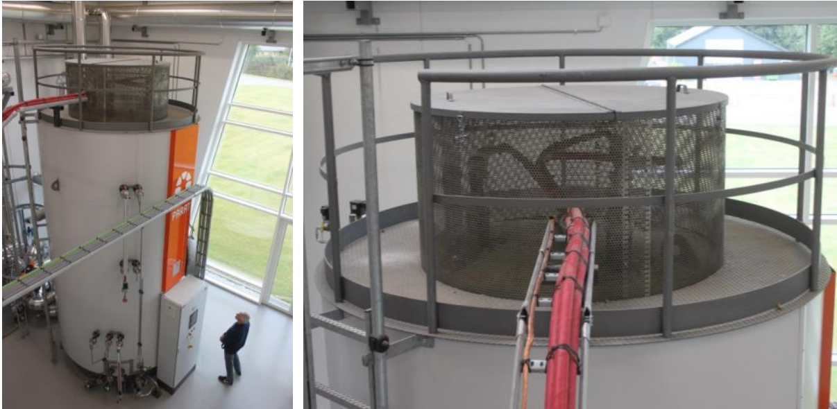
Figure 33: Electric boiler of 10 MW and 14.4 m 3 capacity of the solar district heating plant in Gram, Denmark (Source: Rutz D.)
