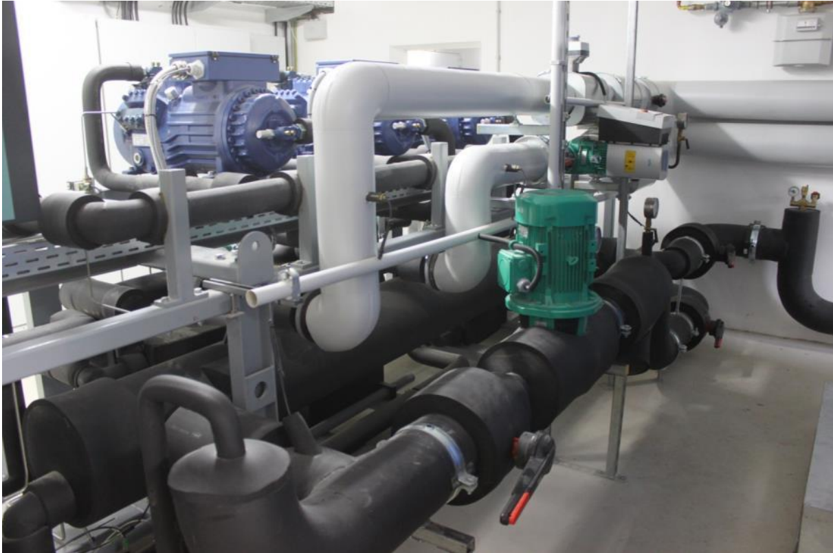
Figure 34: 440 kW ground water heat pump in the small solar heating grid of Dollnstein, Germany (Source: Rutz D.)
