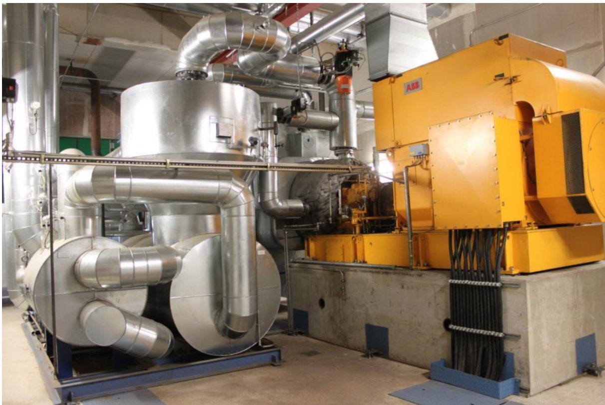
Figure 20: ORC system (1,520 kW el ) of the Grünfütterrocknungsgenossenschaft Kirchdorf a.H. eG in Germany (Source: Rutz D.)
