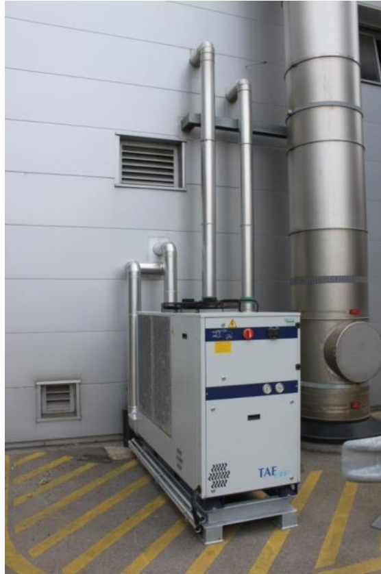
Figure 68: Air-cooled chiller using waste heat of an incineration plant in Austria (Source: Rutz D.)
