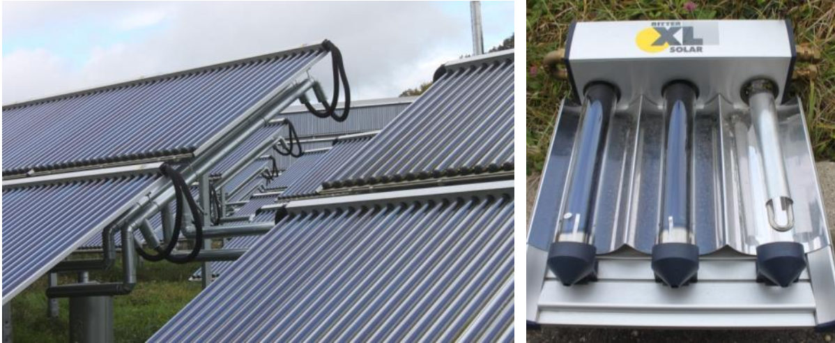
Figure 7: Ground-mounted vacuum tube collectors (left) of the solar district heating plant in Büsingen, Germany and sample of these collectors (right) showing the U-type fluid pipe in the right tube as well as the Compound Parabolic Concentrator (CPC) technology (Source: Rutz D.)
