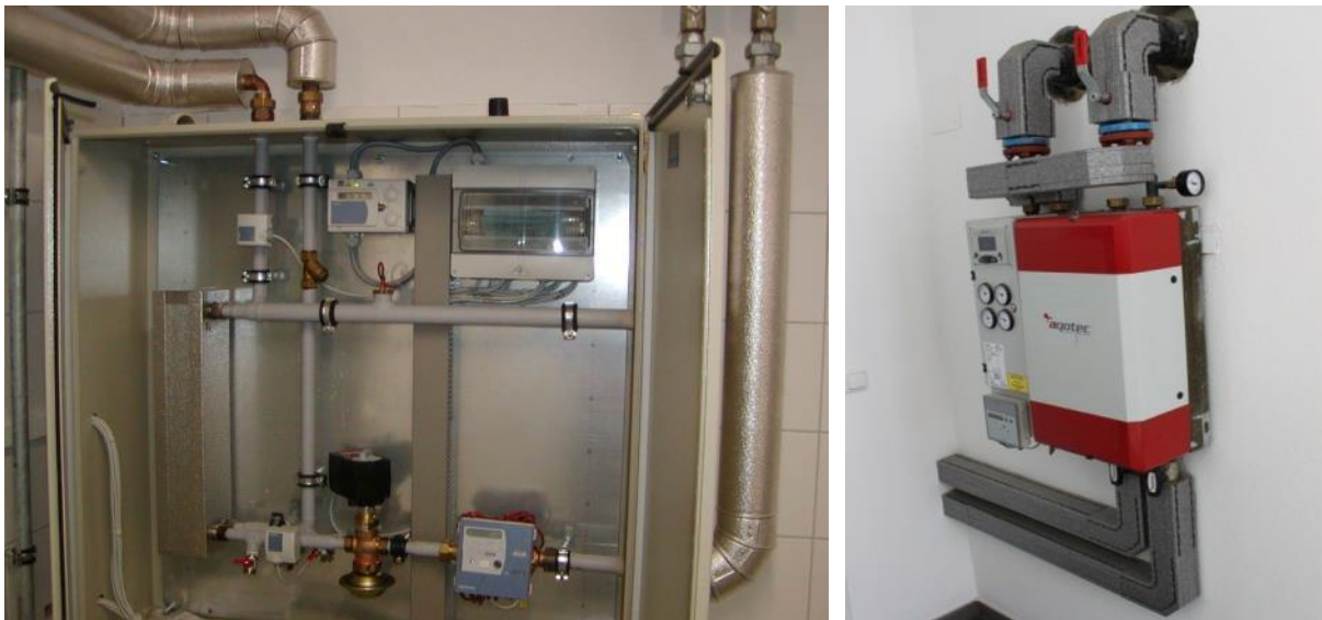
Figure 55: Heat transfer station with a heat exchanger, control unit, valves and a heat meter (left) (Source: Güssing Energy Technologies) and heat transfer station (including a heat exchanger) of an end consumer in Achenal, Germany (Source: Rutz)
