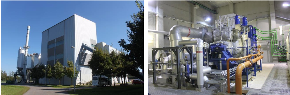
Figure 19: Wood chip fired CHP plant and its steam turbine of the Stadtwerke Augsburg Energie GmbH in Germany (capacity: 80,000 t/a wood chips; 7.8 MW el ; 15 MW th ) (Source: Rutz D.)
