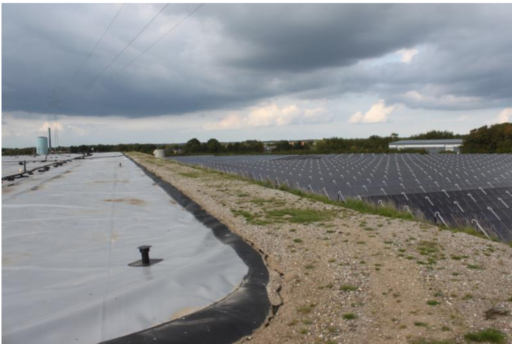
Figure 45: Border of a pit thermal energy storage of the solar district heating plant in Gram, Denmark (Source: Rutz D.)
