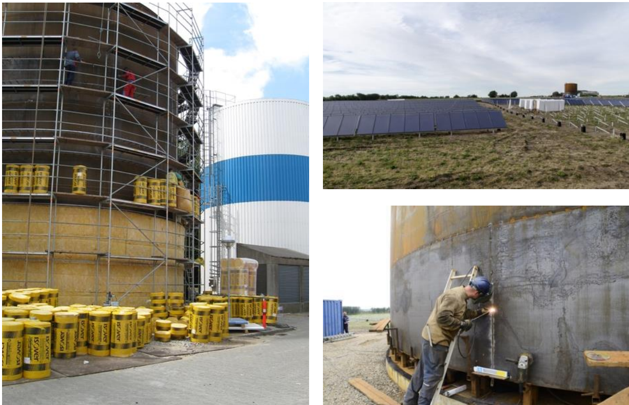
Figure 43: Establishment of steel tanks at Hjallerup District Heating. Left: Establishment of two new steel tanks in connection to the CHP plant in Hjallerup. Right: Establishment of a new steel tank in connection to the solar field and straw boiler. See more about Hjallerup DH in the Best Practice report of Laurberg Jensen et al. (2016) (Source: www.hjallerupfjernvarme.dk )
