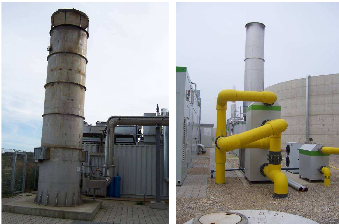
Figure 7.28 Modern biogas flares (RUTZ 2007)
