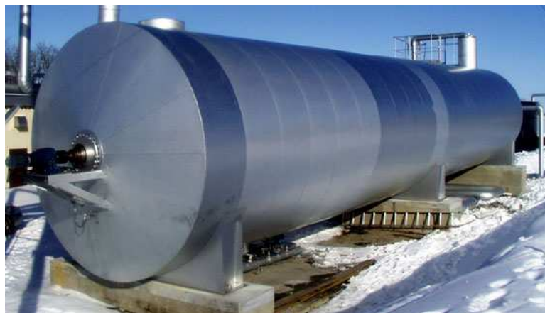
Figure 4.3 Horizontal digester, built in Denmark (Nordisk Folkecenter 2001)
