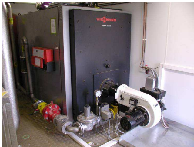
Figure 5.2 Biogas burner for heat production (AGRINZ 2008)
