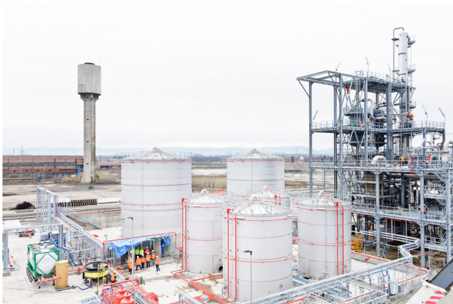
Figure 31: Ethanol Storage and distillation area
