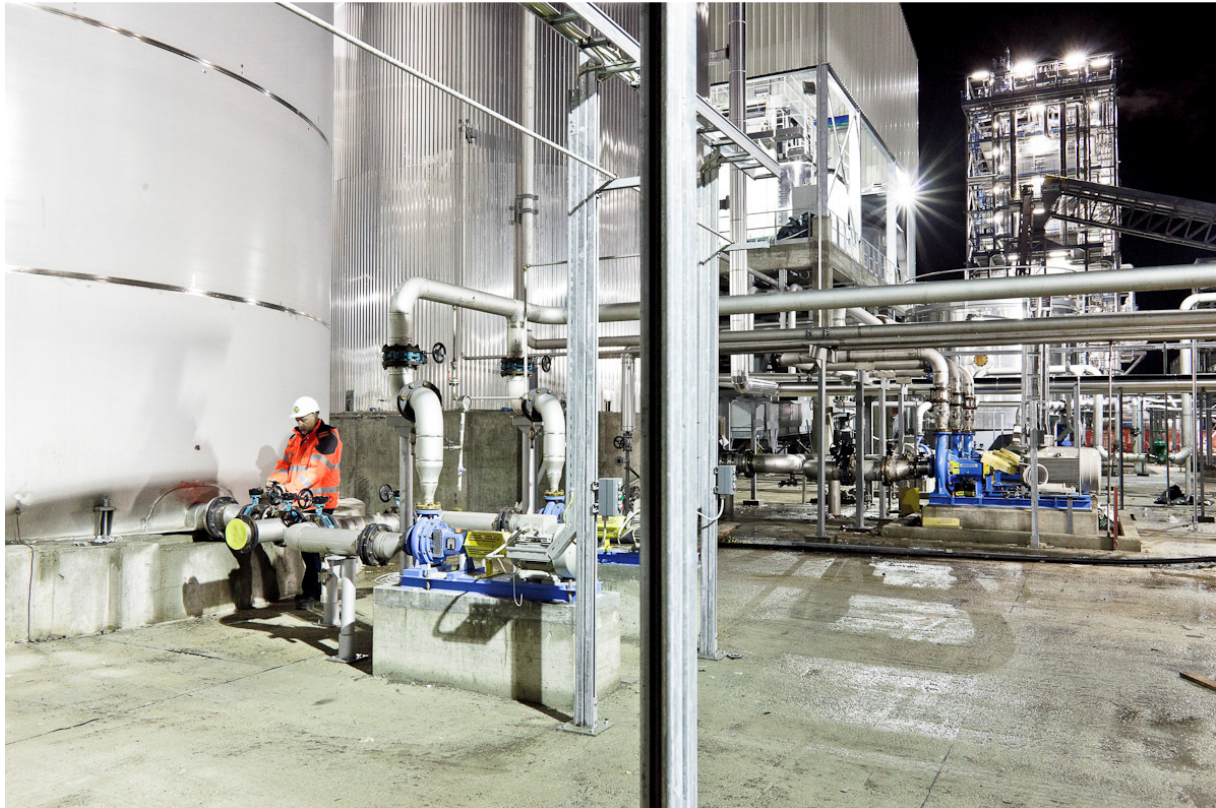
Figure 1: Night view of Crescentino ethanol plant
