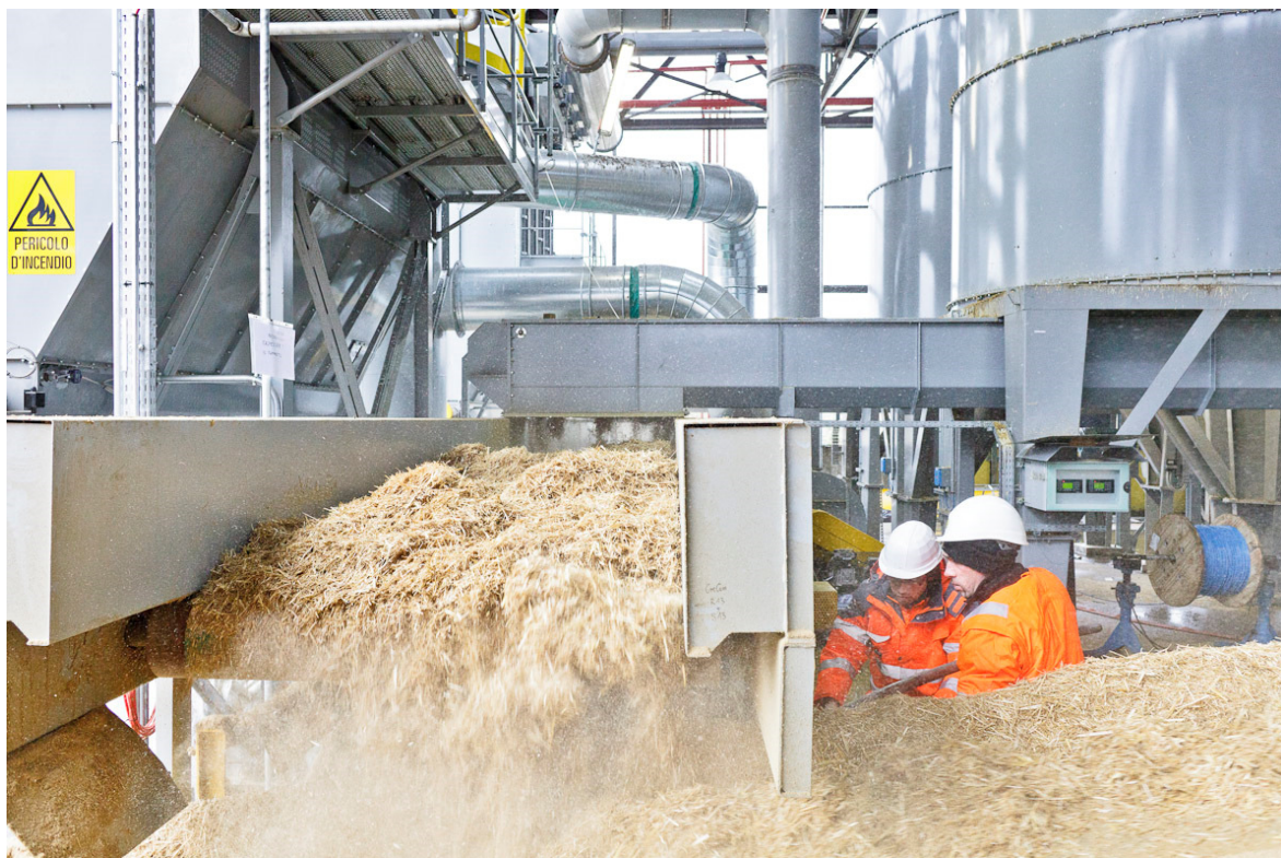
Figure 14: The conveyor system after the debaling
