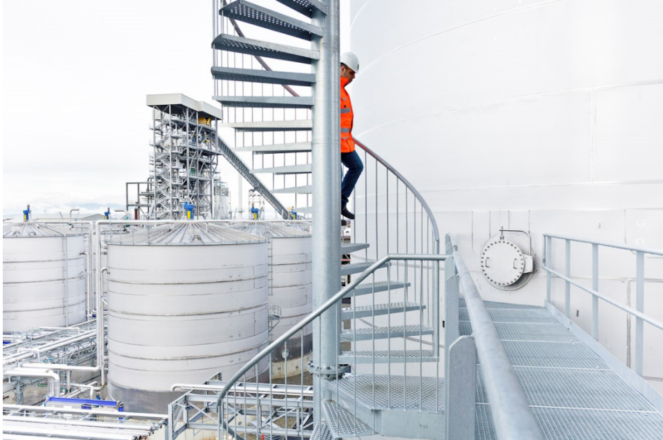
Figure 19: The pretreatment area behind the fermenters
